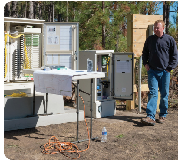
CTC working in the field at the area cabinet.
