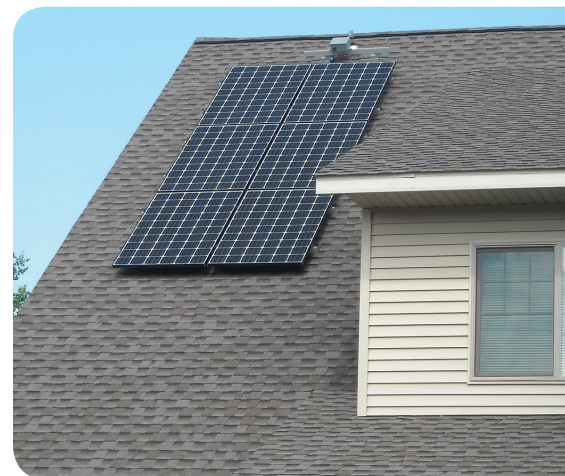
Close-up of the Photovoltaic panels on the roof of Sprucewood Townhomes.
